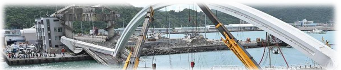
Traditional structure coating degrades under outdoor UV exposure and allows penetration of moisture with salt ions and corrosive gases such as H 2 S, SO 2 , etc. to cause structural corrosion and degradation of structural integrity and loss of lives and properties.
