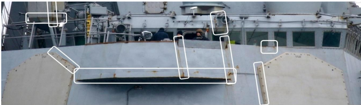
Figure 9: The above public picture depicts excessive corrosion of the USS ARLEIGH BURKE DDG51 in the Black Sea in 2021. The highlighted areas of excessive corrosion are mostly at the edges and corners where stresses tend to concentrate to cause the protective paints failure to allow moisture laden with dissolved salts to get into the interfaces between steel and coating.
