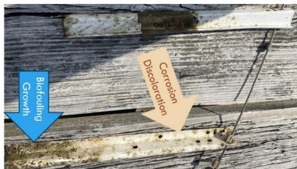
Figure 15: The top piece of epoxy coated steel coated with field applicable PVDF after 30 days submersion in Chesapeake Bay, Maryland during the month of June. The cut edge showed corrosion and initiated with some biofouling growth and starting to migrate to the other edge. The bottom piece of the other half of epoxy coated steel without PVDF top coating showed substantially more biofouling growth along with more obvious brownish corrosion coloring.
